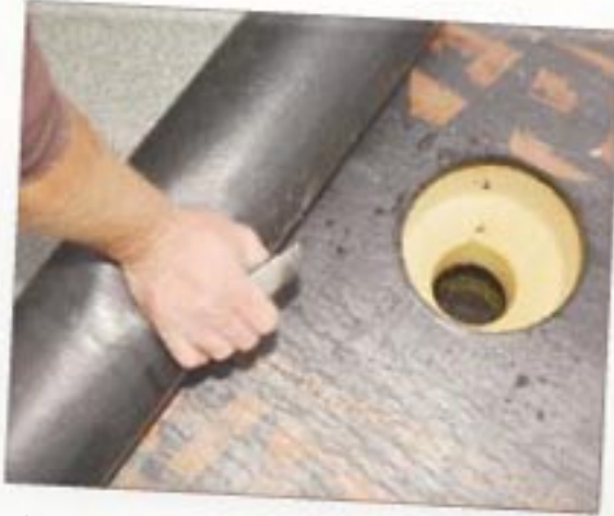
The final lap. Important – the hole for the drain also needs some attention.
