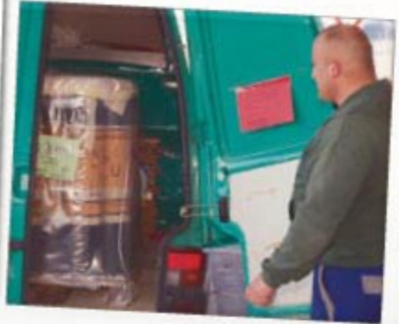
... the first layer of the new roof is already on the way.
