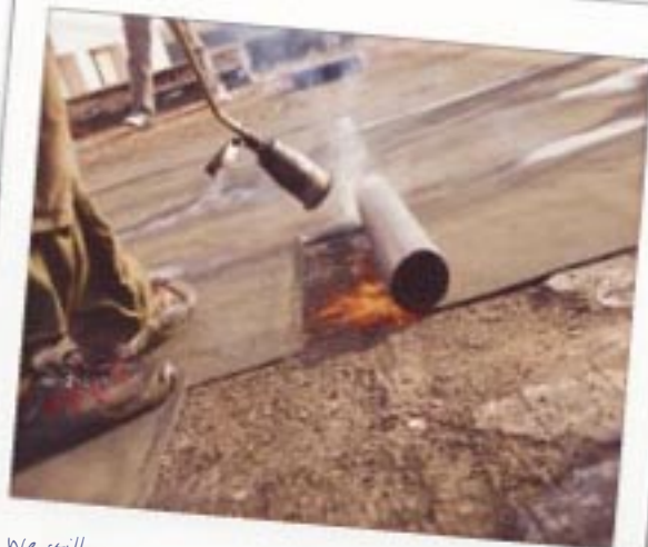
We still manage to install the first sections of the vapor barrier on the bare roof before the end of the day.
